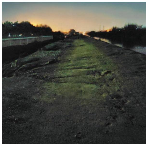
A stretch of road in Bawana with poor lighting
